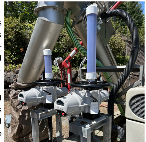
Newly Installed Actuator Motors
